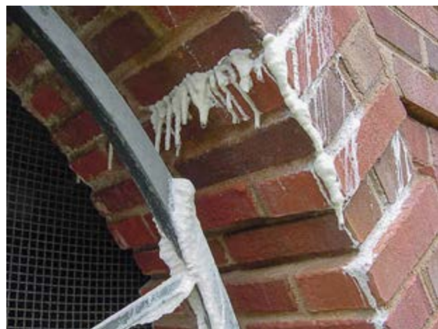
Lime run and calcium deposits on brick
