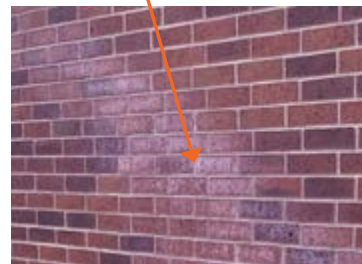
Hard water deposits on brick
