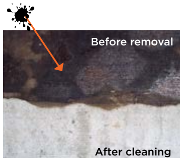
Oil on concrete
