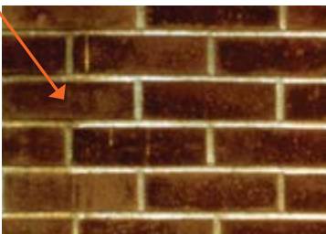
Acid burn on brick
