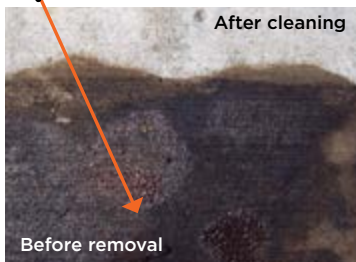
Oil on Concrete
