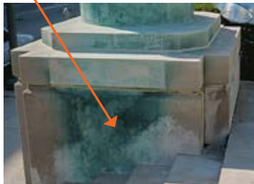
Copper staining on concrete
