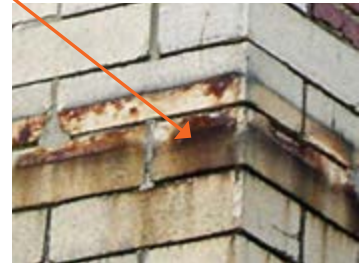
Rust on fired brick
