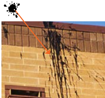
Tar on brick
