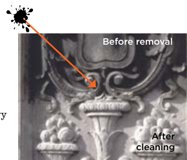
Carbon staining on limestone
