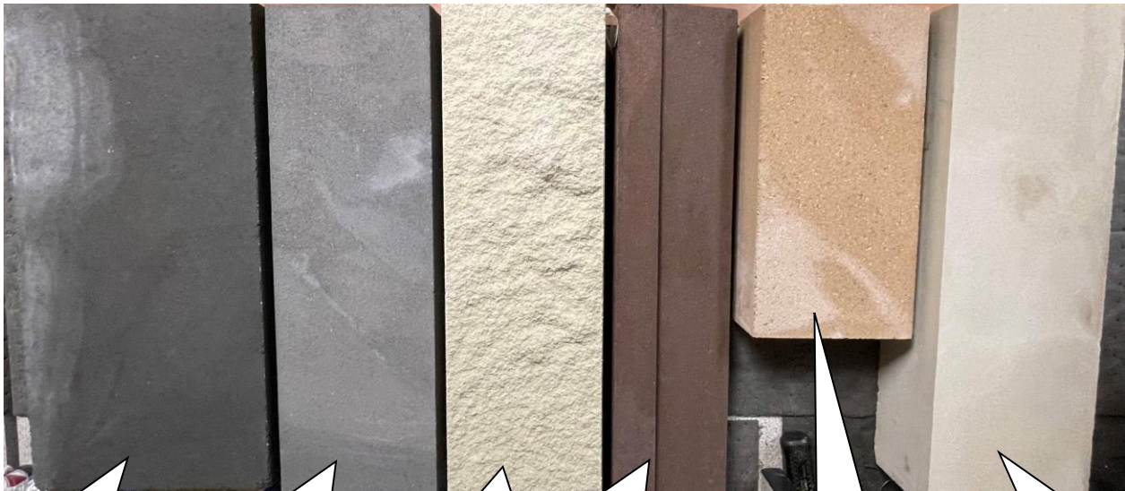
Efflorescence Staining Present on Samples as Submitted
