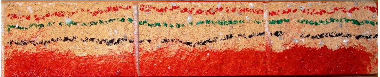
“Marigold Split Face CMU; Before Graffiti Removal
