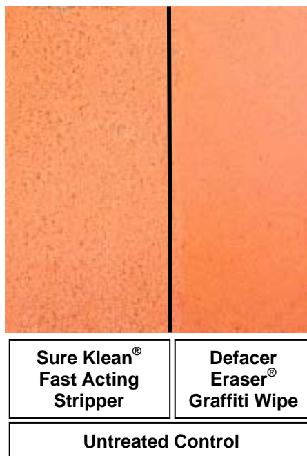
“Sedona Clay – Astra-Glaze-SW+®” Glazed CMU; After Graffiti Removal
