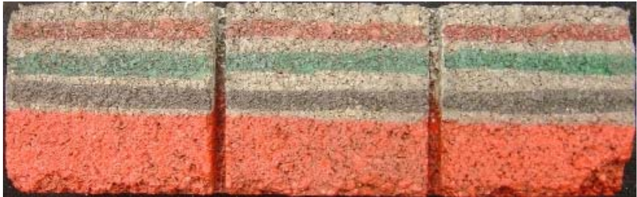
“Leatherwood” Concrete Brick; Before Graffiti Removal
