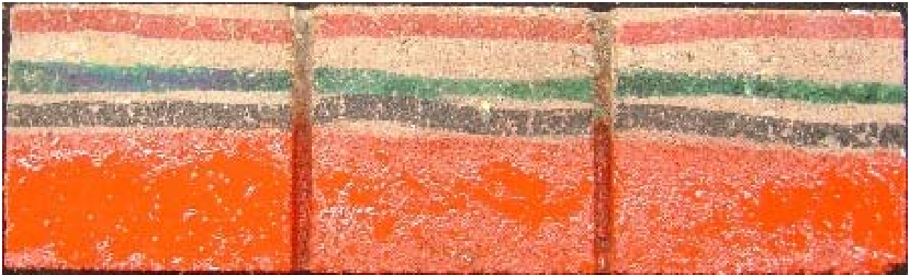
“Red Clay” Concrete Brick; Before Graffiti Removal
