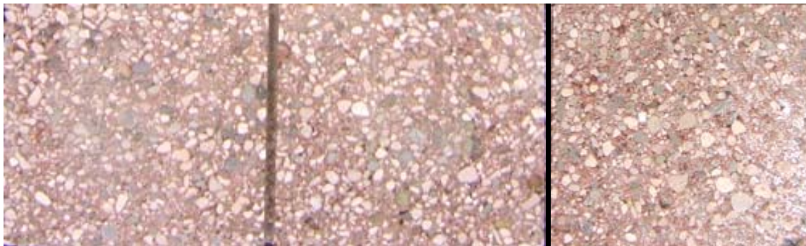
Sure Klean® Burnished Custom Masonry Cleaner (1:2) Sure Klean® Burnished Custom Masonry Cleaner (1:3) Un-cleaned
