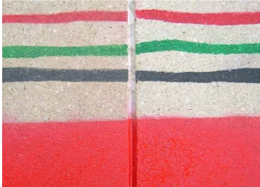
“WC1090”; Before Graffiti Removal
