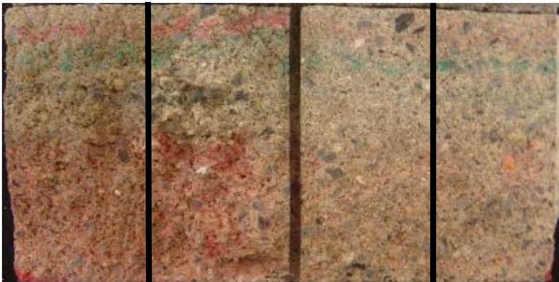
“#7 Lt. Wt.” Split-face CMU; After Graffiti Removal
