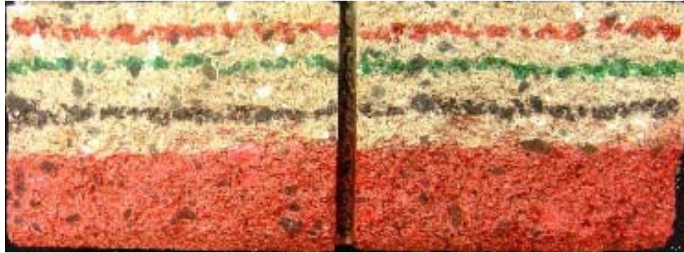
“VL Tan” Split-face CMU; Before Graffiti Removal
