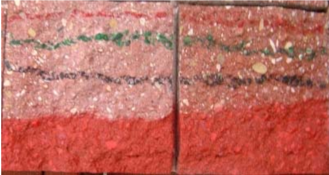
“5558” Split-face CMU Before Graffiti Removal
