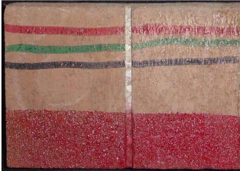
“Red Quick-Brick” CMU Before Graffiti Removal
