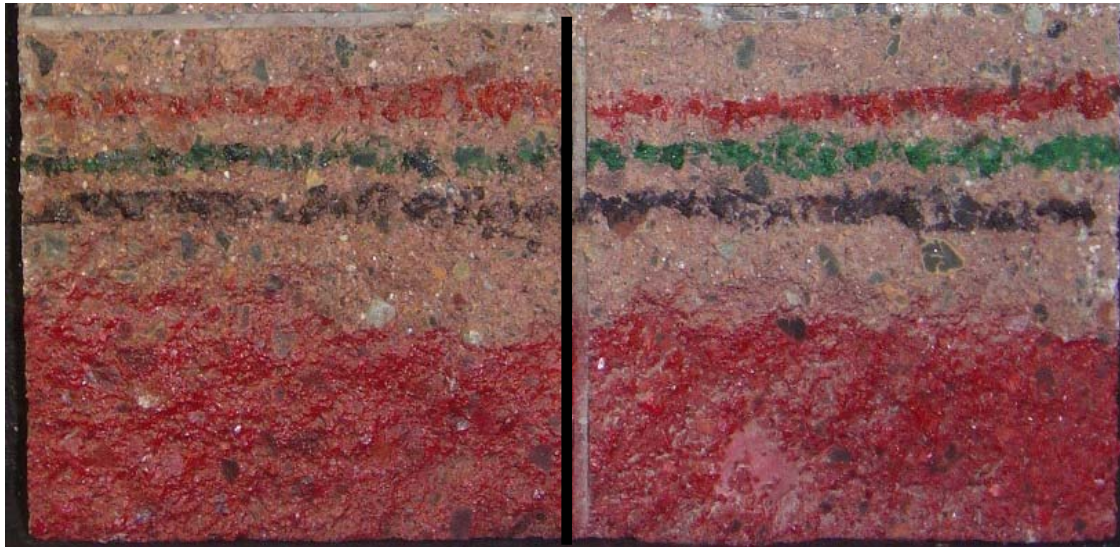
“869 (Red)” Split-face CMU Before Graffiti Removal
