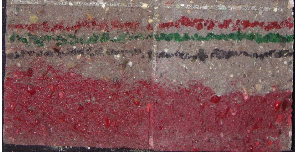
“3” “Dark Brown” Split-face CMU Before Graffiti Removal
