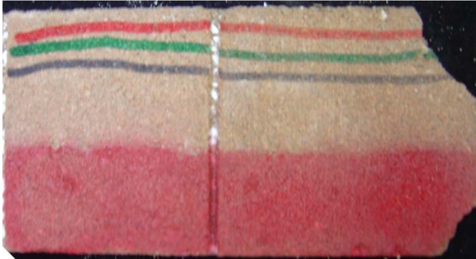
“Gold” Smooth-face Concrete Brick Before Graffiti Removal
