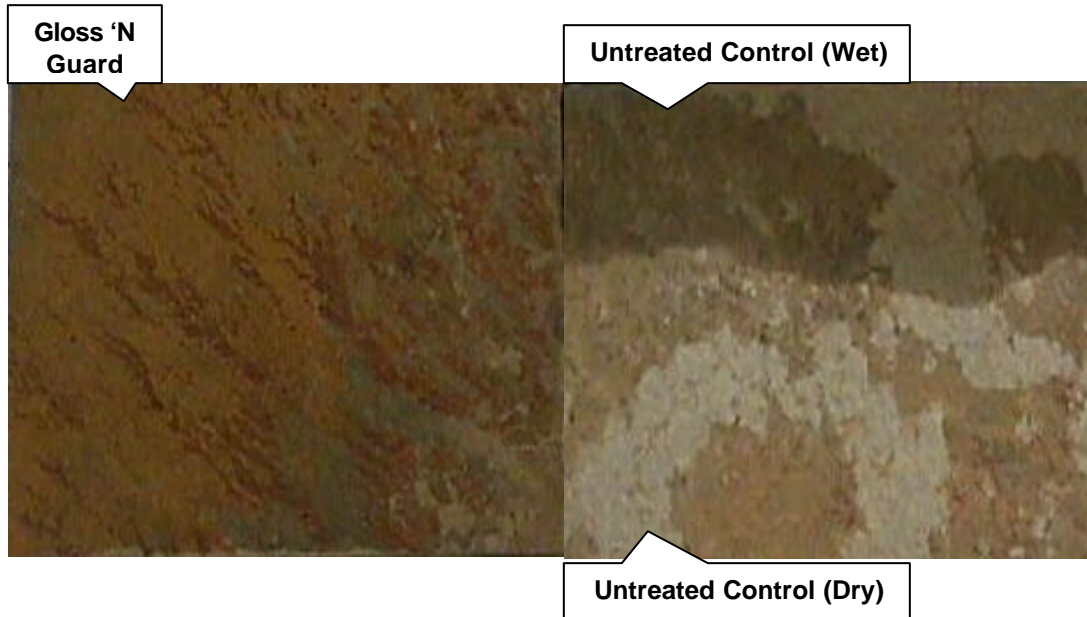
PHOTO C – “Gray/rust” slate tile after color enhancement
